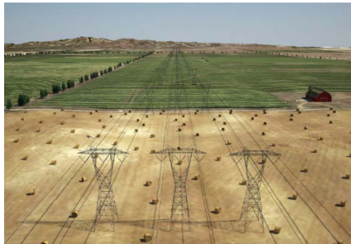
Three 500 kV lines 600 foot ROW
